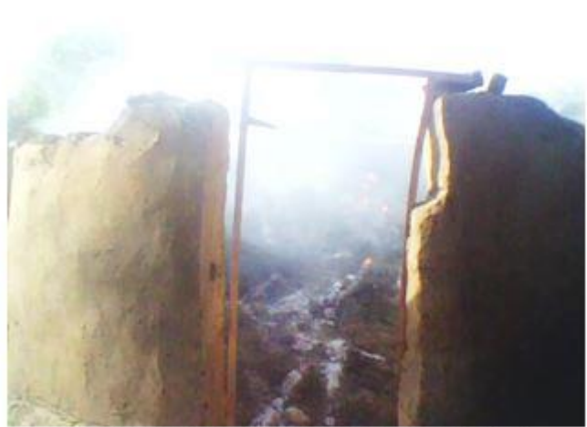
A house that was completely burnt in fire incident
