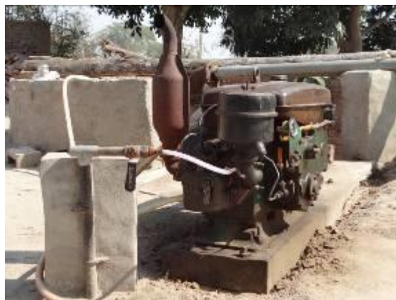
16 Horse Power Diesel-Engine Shifted on Biogas
