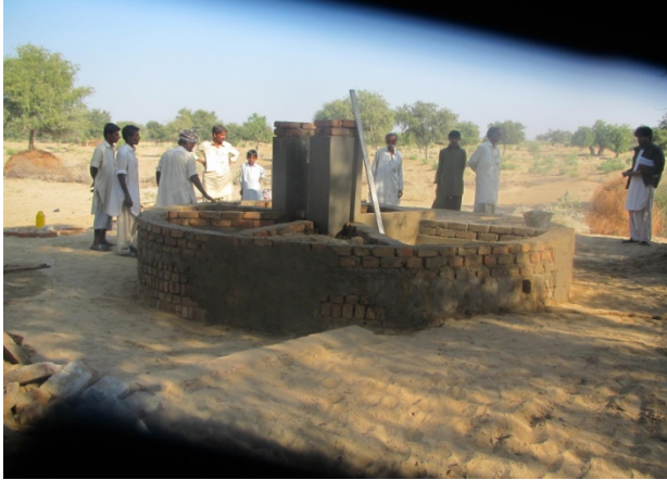
Work in progress on repairing of a dug well in VDMC Lakhmia District Tharparkar
