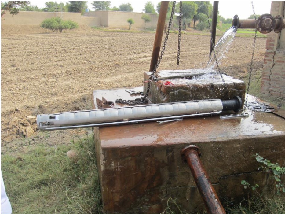
Water coming from the scheme
