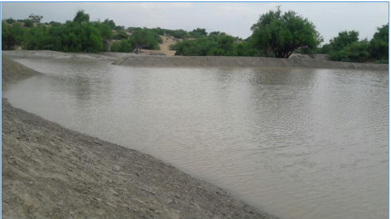
A natural depression (locally known as Tarai) rehabilitated at district Tharparkar. The structure collects and store rain water for long period.
