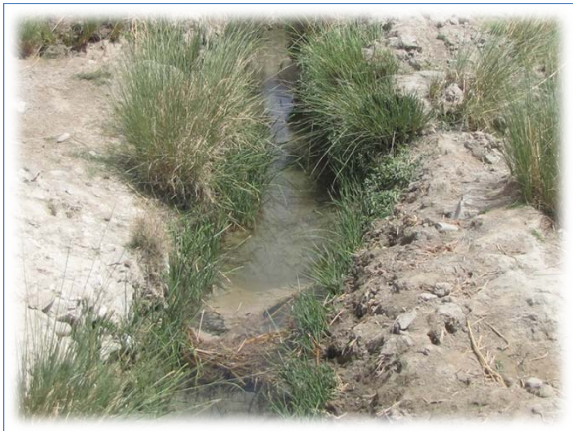
Figure 79: The condition of the water delivery channel at Qila Iskan Khan
