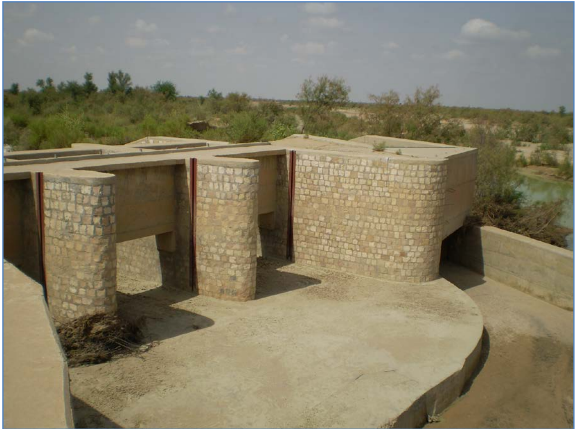
Figure 21: Weir, upstream view of sediment sluice of the Chandia Spate irrigation scheme, Sibi district, Balochistan, Pakistan
