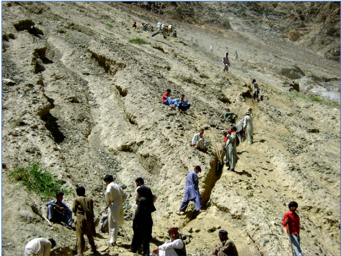
Figure 16: WUA members involved in earthwork at High Pressure PE Pipe Irrigation System at Nomal, Gilgit
