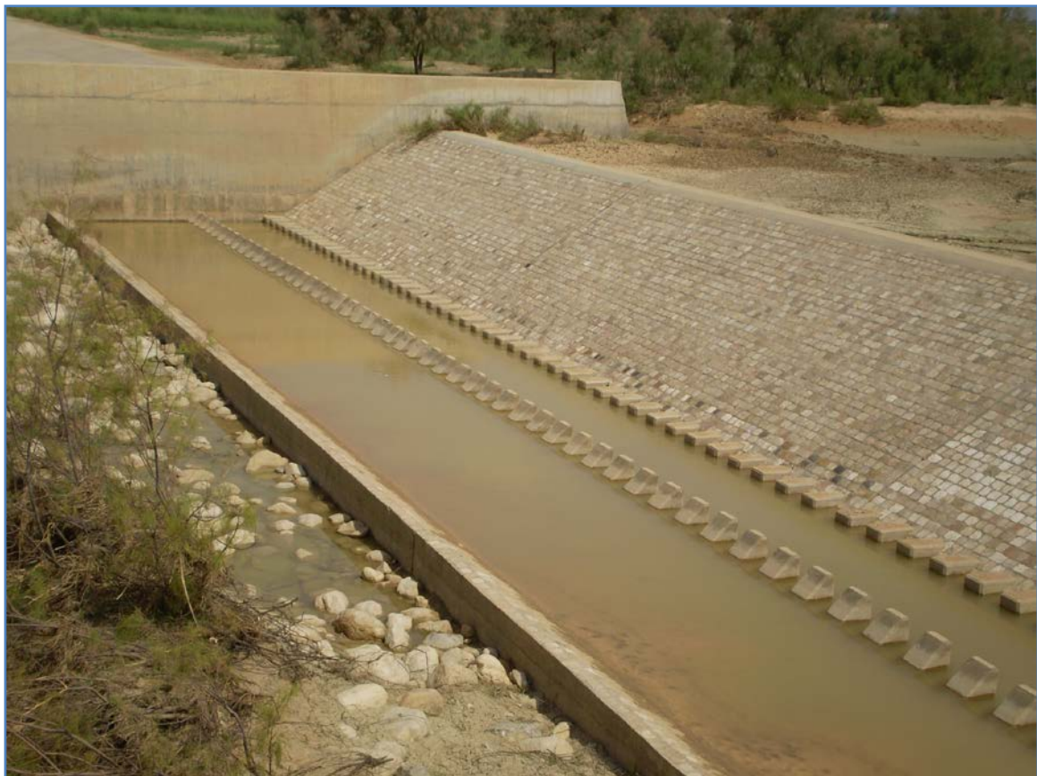
Figure 20: Weir, upstream view of head regulator of the Chandia Spate irrigation scheme, Sibi district, Balochistan, Pakistan
