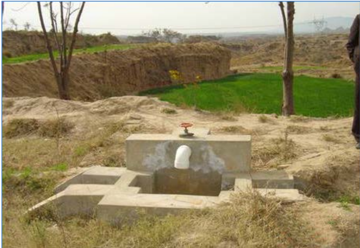
Figure 35: Mini dam structure and command area with pipe-flow irrigation system
