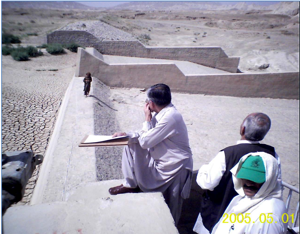
Figure 22: Weir structure and head regulator at Shabo Headworks, Pishin district, Balochistan, Pakistan
