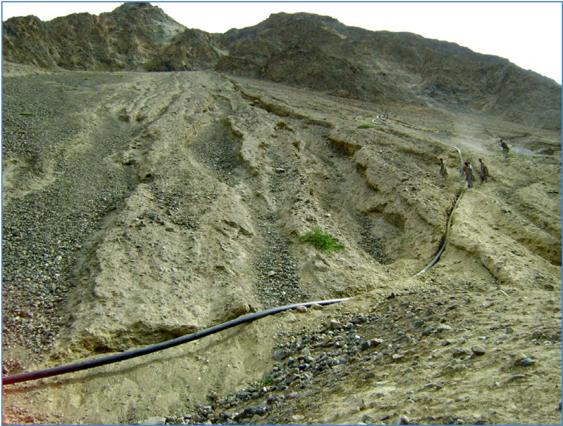
Figure 17: WUA involved in laying of PE High Pressure Pipe under the supervision of Dadex Eternit Pvt Ltd., WMD-AD and NESPAK Engineers at Turmai High Pressure PE Pipe Irrigation System at Nomal, Gilgit
