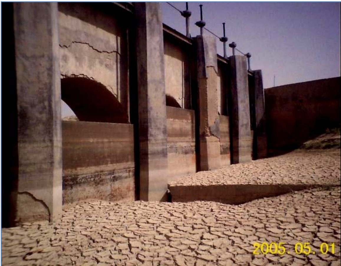
Figure 26: Gated weir controlled off-stream water diversion to water tanks
